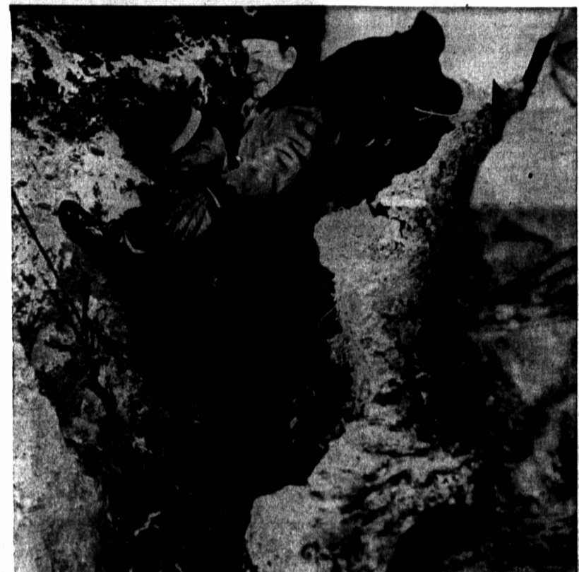
CNST. BOB WILLIAMS of the R.C.M.P., and Cnst. Elmer Martin of the Summerside Police Department, are seen working in the six-foot trench to recover the body of Mr. Clements who had been in a crouched position lying pipe when the cave-in occurred. Photo by Wollan.
