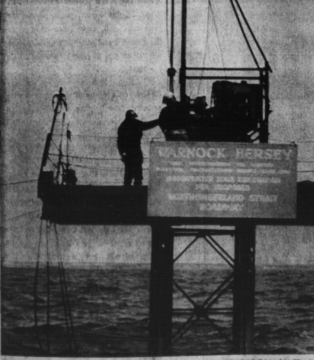
A CREW FROM WARNACK HERVEY SOIL INVESTIGATIONS LTD. DRILLS INTO BEDROCK FOR A NINE-MILE CROSSING OF NORTHUMBERLAND STRAIT. THE TEST BORINGS ARE A FIRST STEP IN THE FULFILLMENT OF A PLAN TO CON-
